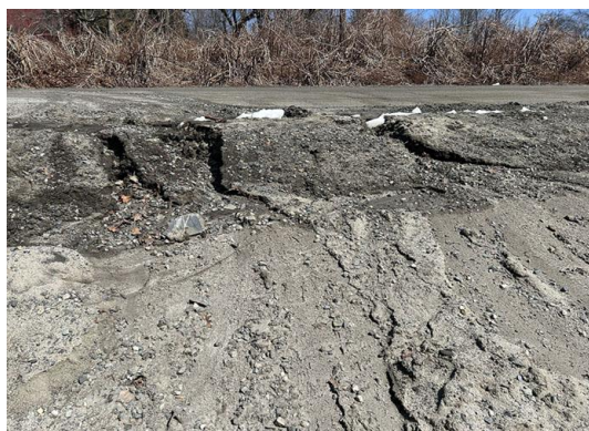
After cutting JK, erosion shows
