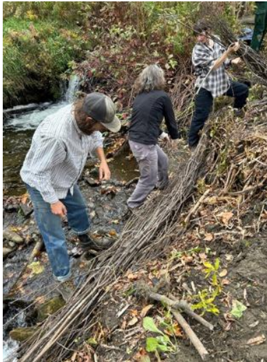
Farley Brown's Watershed Class staked non-growing fascines on the 4' high stream bank to give more stabilization to the bank over the winter.
