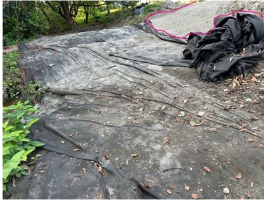
9/17 The area outlined in red shows where rocks were removed and the gully filled. The whole road bank with its many gullies had the same treatment.
